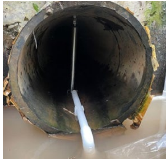
AVFM 6.1 sensor monitoring flow at pipe outlet.
