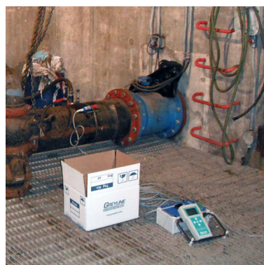
Greyline PDFM 5.0 Portable Doppler Flow Meter With Ultrasonic Sensor on 12" Sewage Forcemain
