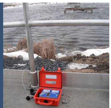
Stingray Ultrasonic Sensor installed in North Glengarry 16" sewage lagoon inlet
