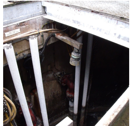
A typical wet well application.
