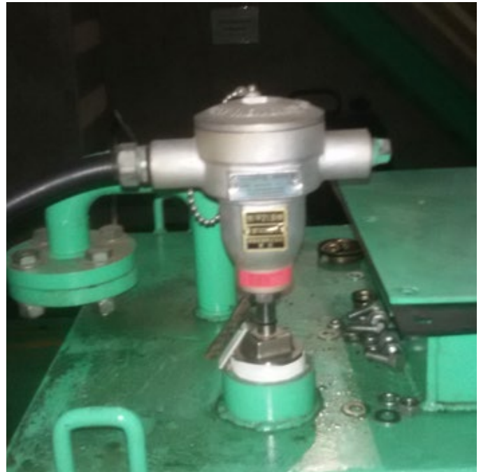
A Pulsar Measurement dB10 transducer on site at a chemical plant in Thailand.
