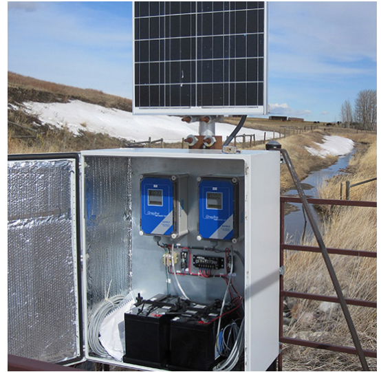
Greyline AVFM flow meter electronics installed in solar-powered panel
